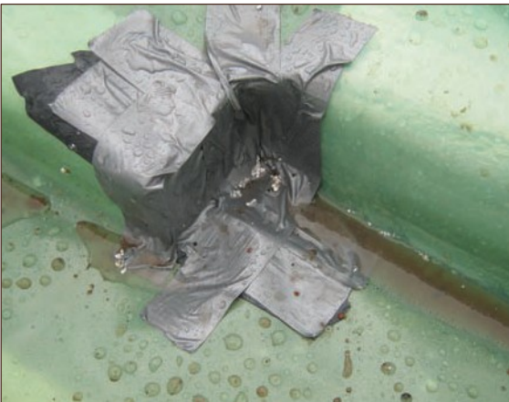
Figure A4.69 Attempt at corner detailing using non-proprietary duct tape (courtesy Smith Grant)
