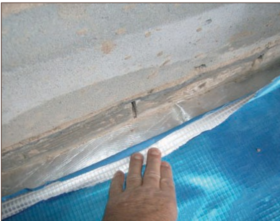
Figure A4.77 Small lap and no single sided tape used to achieve secondary seal (courtesy Smith Grant)
