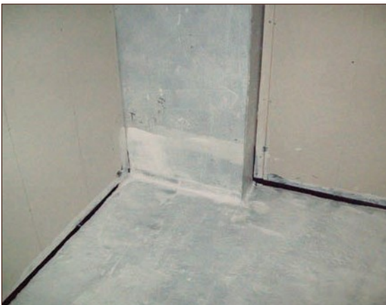
Figure A4.83 Poor quality installation of liquid gas membrane. Liquid gas membranes come in two colours (black and white) allowing coverage of each coat to be easily assessed. Here the gas membrane has been spread too thinly and inconsistently. In addition, it appears to have been applied to a damp surface, causing blistering (courtesy Card Geotechnics Limited)
