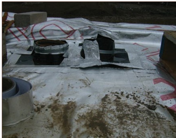
Figure A4.72 Joint between top hat and gas membrane has lifted due to poor fit and attempt to construct in very wet conditions (courtesy Smith Grant)
