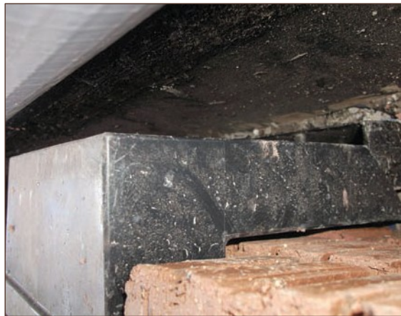
Figure A4.88 Ventilator becoming detached to fit to external block work. This is due to builders requiring increased cavity widths to achieve thermal properties expected by Building Regulations (courtesy NHBC)
