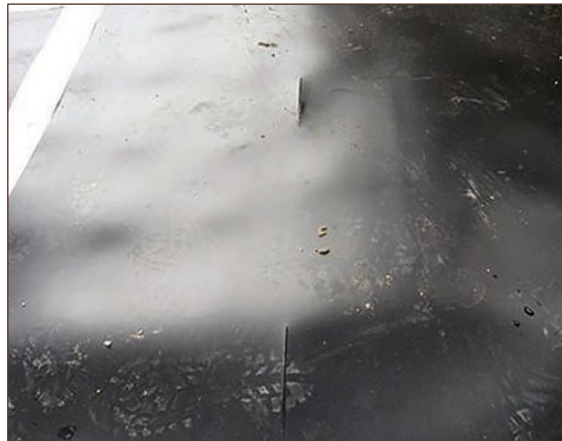
Figure A4.58 Damage caused to gas membrane by follow-on trade who cut/shaped the dry lining board directly on the unprotected installed gas membrane (courtesy NHBC)
