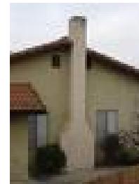
Example of an external Chimney
