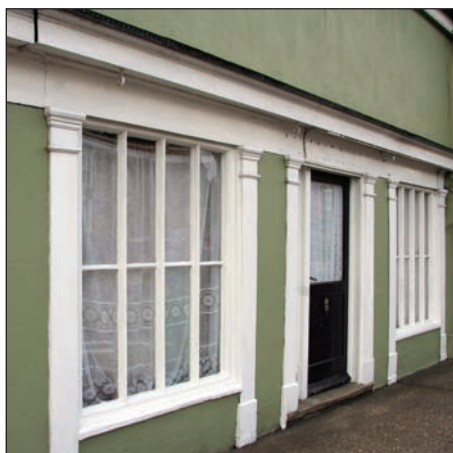
▲ 13 Victoria Street retains a fine example of a mid C19 shop front.
