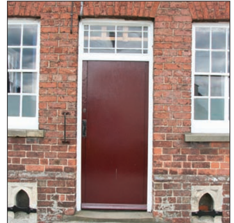
▲ The mid C19 door to the Baptist Chapel. Over the door is a margin light fanlight, a feature found on other buildings of similar date in the village.
