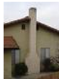
Example of an external Chimney
